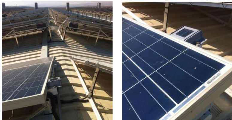
Figure 9: Irradiance sensors installed in line with the monitored array
