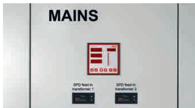
Visual indicator for surge protective devices installed in switchgear cabinets.
