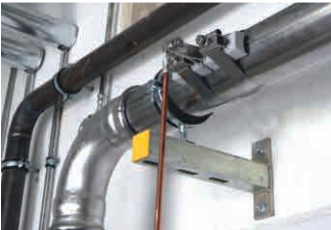
Installed at a StSt pipe.
