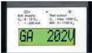
Indication of the measured sparkover voltage.
