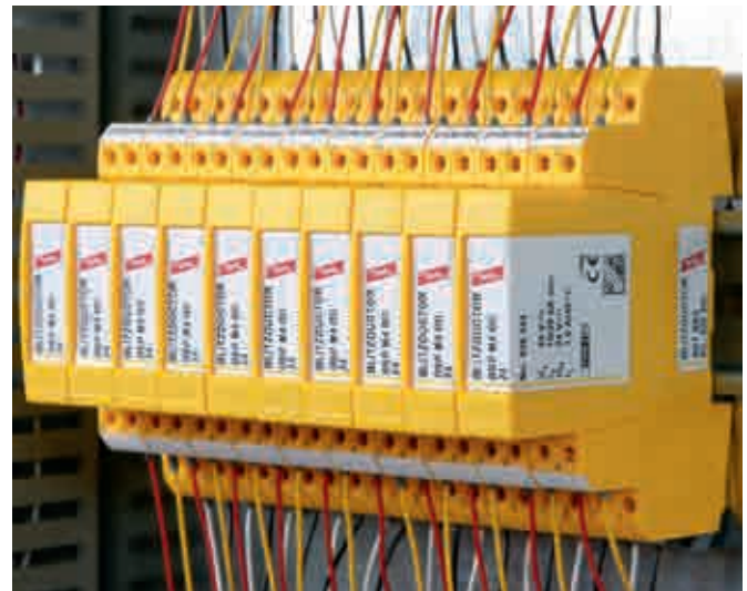
Pluggable and universal multipole surge arrester for use in information technology systems.
