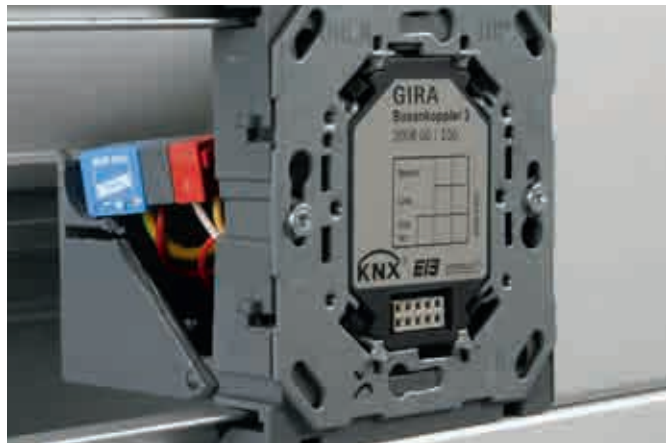
Protection of a KNX bus coupling unit by means of a BUSstector surge arrester mounted on a bus terminal in the mounting panel of a cable duct.
