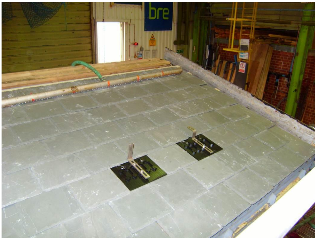
Figure 1 A general view of the test rig showing the installed Solar Slate Plates
