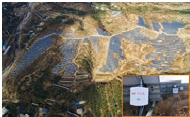
Liaoning Jiuzhai Gaizhou PV plant 20MW
