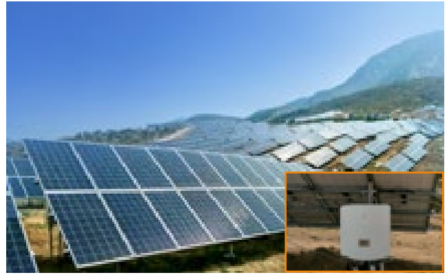
Liaoning Yingkou Jiuzhai PV plant 20MW
