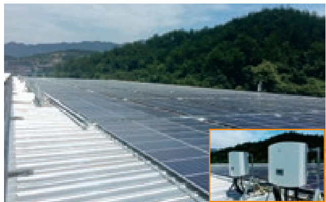
Hainan JiuLongGlass 1.7MW
