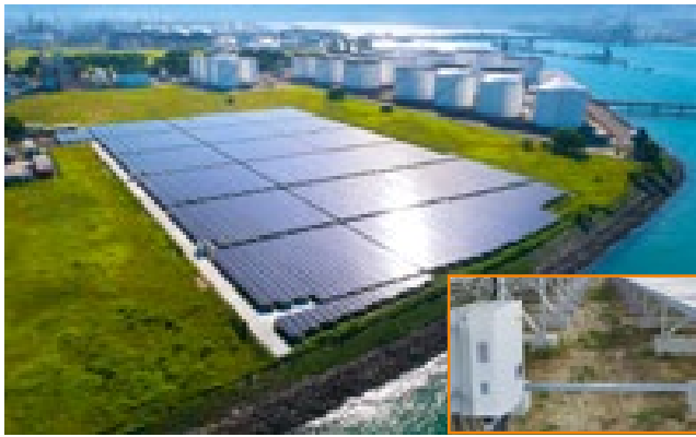
JTC Solar Farm, Singapore 5MW
