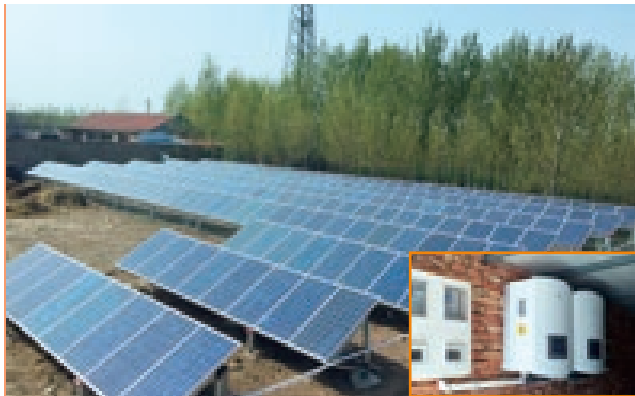
Shandong Leling poverty alleviation PV Plant 50kW
