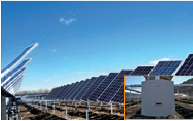
Hebei Zhangbei Agricultural-photovoltaic hybrid PV plant 50MW
