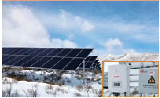
Shanxi Guangling PV plant 1.47MW
