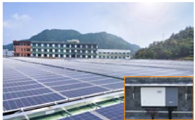
Tyco Electric, Panan Jinhua Zhejiang 1.5MW
