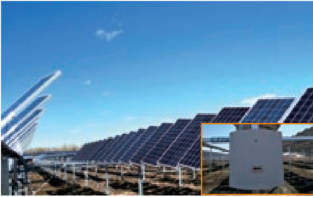
Hebei Zhangbei Agricultural-photovoltaic hybrid PV plant 50MW
