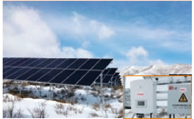
Shanxi Guangling PV plant 1.47MW
