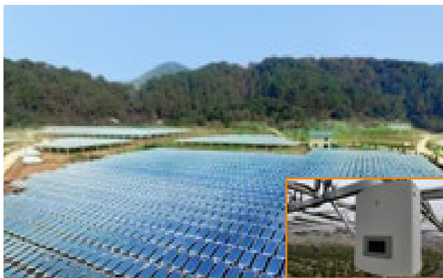
Zhejiang Dajie Agricultural-photovoltaic hybrid PV plant 3MW
