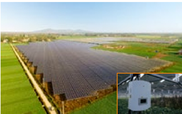
Hubei Guanyin Agricultural-photovoltaic hybrid PV plant 20MW
