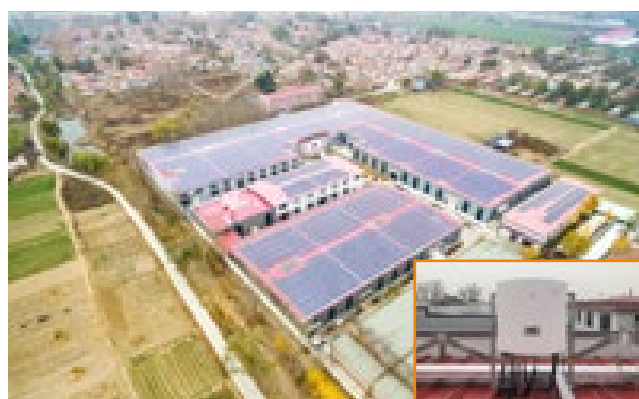
Shandong YUELONG 3.5MW
