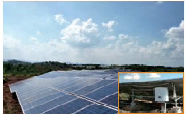
Jiangxi Ganzhou PV Plant 3.5MW
