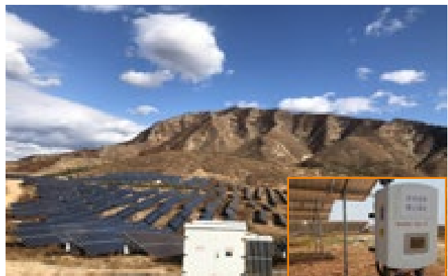
Liaoning Gaizhou Jiuzhai PV plant 20MW
