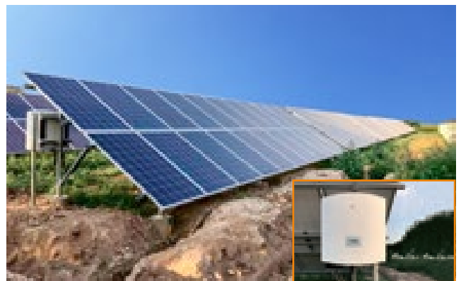
Hebei Qinghuangdao poverty alleviation PV Plant 5MW
