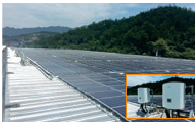
Hainan JiuLongGlass 1.7MW
