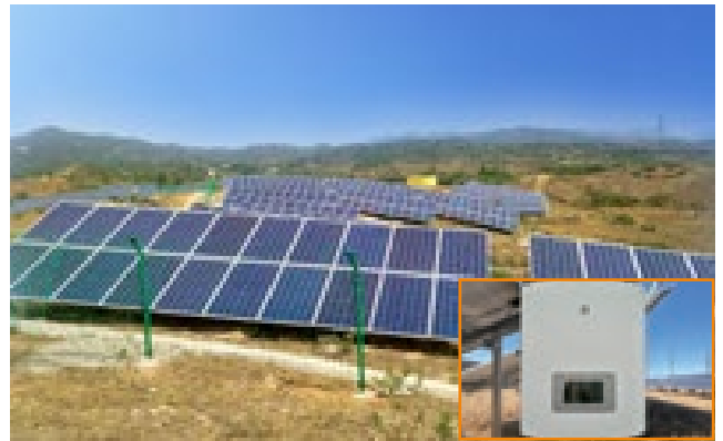
Hebei Qinghuangdao poverty alleviation PV Plant 9.7MW
