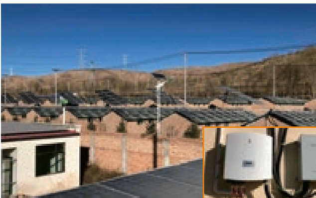
Qinghai HuzhuBanyan poverty alleviation PV Plant 2MW
