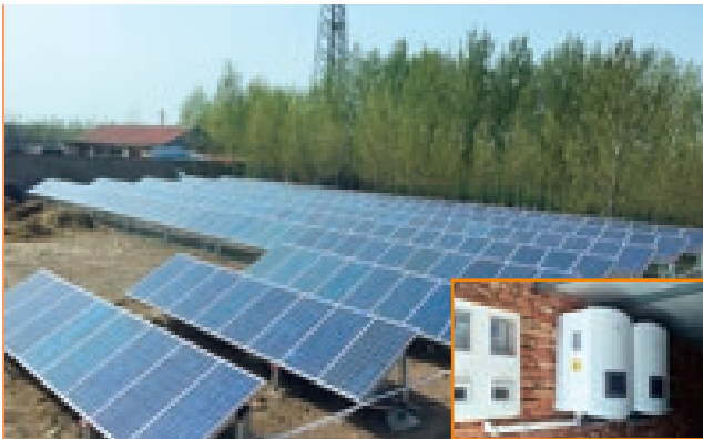
Shandong Leling poverty alleviation PV Plant 50kW
