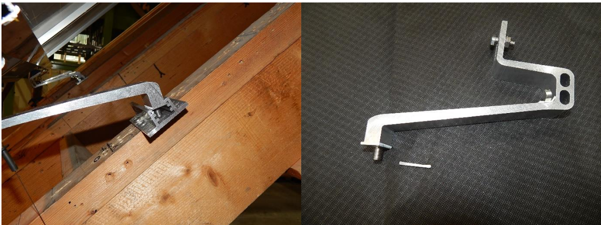
Figure 18. Image to show the ultimate failure of the RH flat roof hook system.
