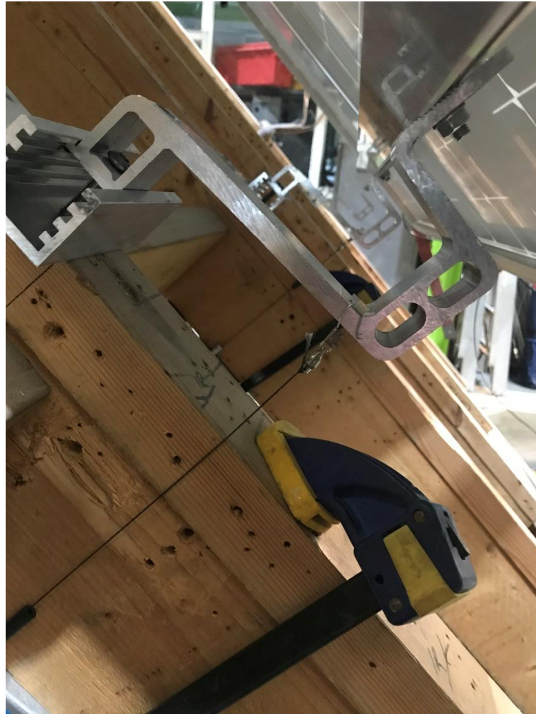
Figure 10. Image to show the installation of a displacement gauge on the RH1 and RH Flat roof brackets.
