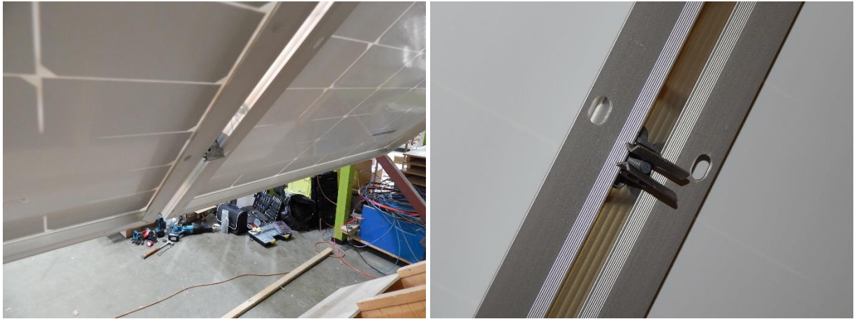
Figure 20. Image to show the ultimate failure of the hanger bolt system.
