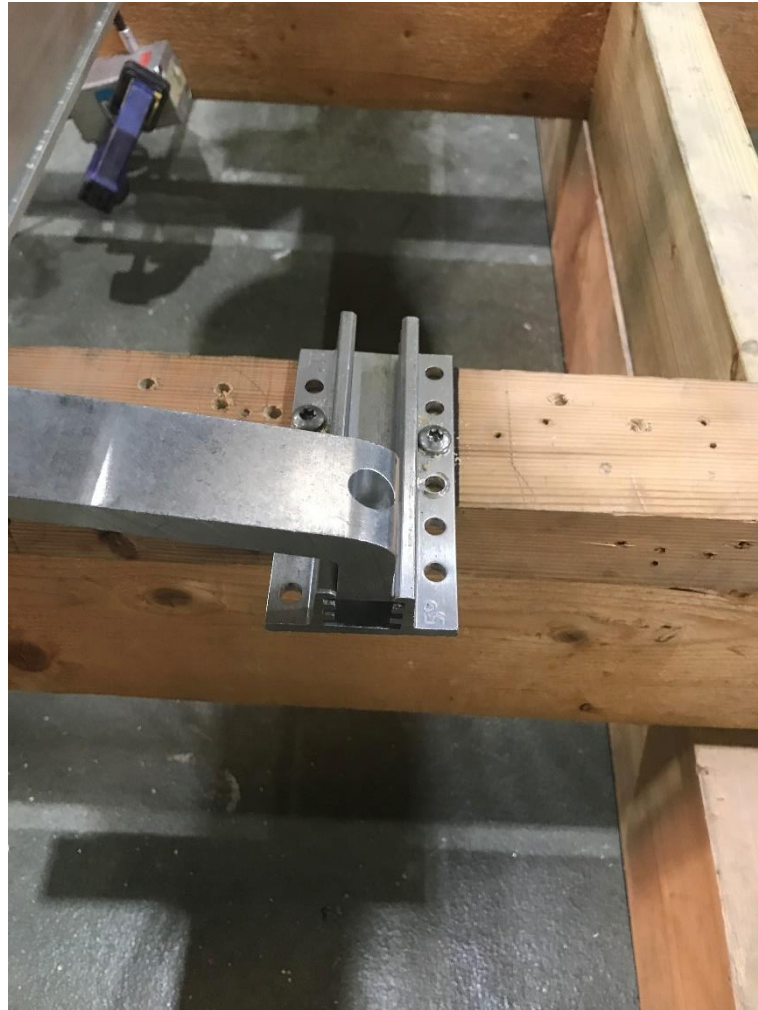
Figure 4. Installation of the RH Flat Roof Hook to the BRE test rig.
