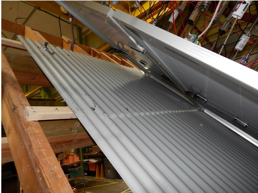
Figure 22. Image to show the ultimate failure of the Metasole bracket system.
