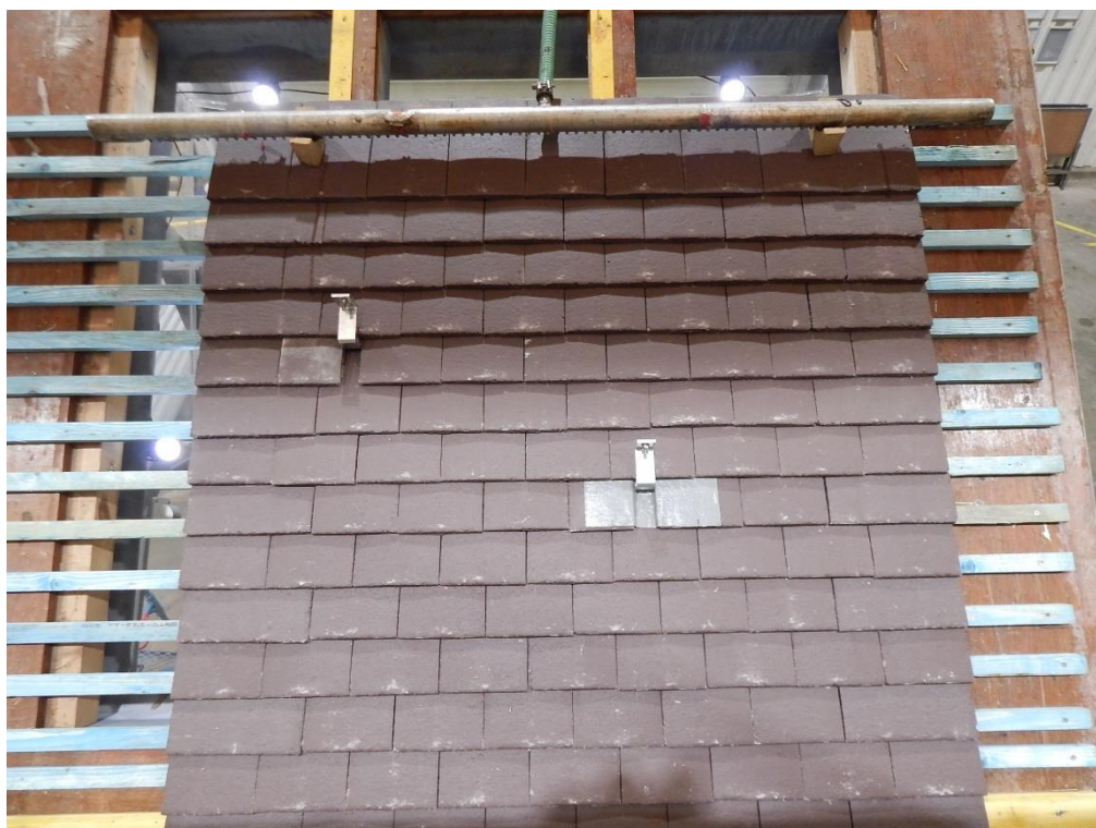
Figure 5. RH flat roof hook installed on the BRE test rig prior to test.
