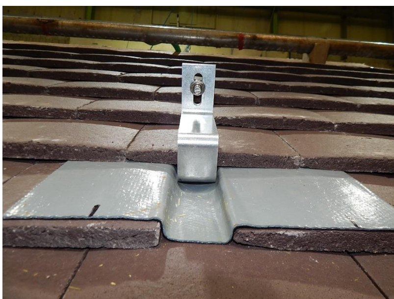
Figure 6. Gap created by installation of the RH flat roof bracket.
