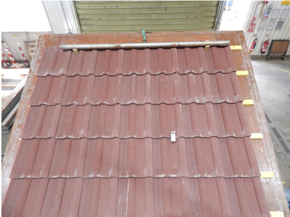
Figure 1. RH1 roof hook installed on the BRE test rig prior to test.
