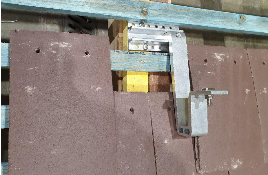
Figure 3. Slot cut out of tiles to accommodate the RH flat roof hook.
