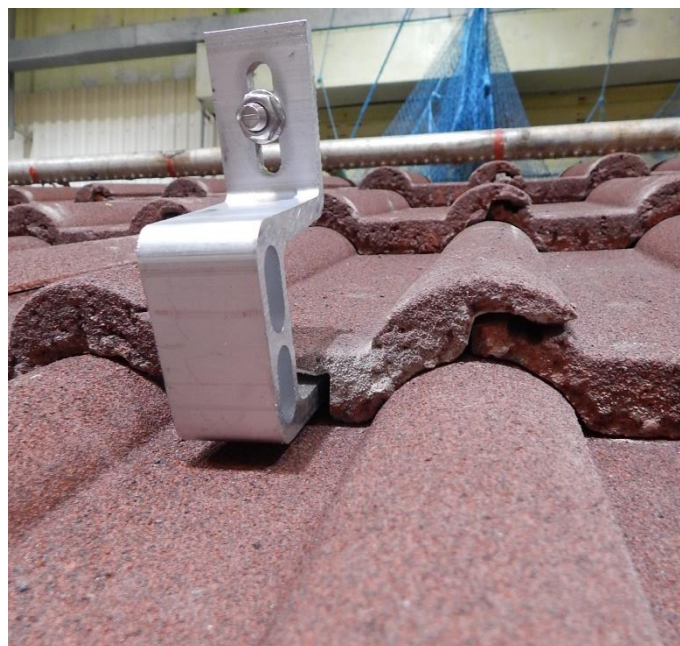
Figure 2. Close up of installation of RH1 roof hook with notch cut out of tile.
