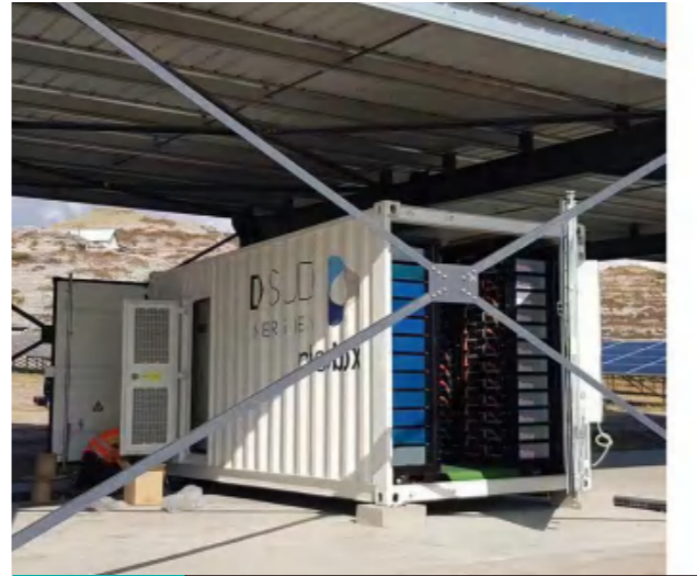
MADAGASCAR 1.5MWH/500KW Micro-grid Self-consumption ESS PV+DG+BESS
