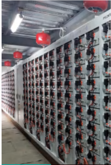
BEIJI Island CHINA 2.65MWH/1.2MW Micro-grid Self-consumption /Back-up ESS PV+DG+BESS
